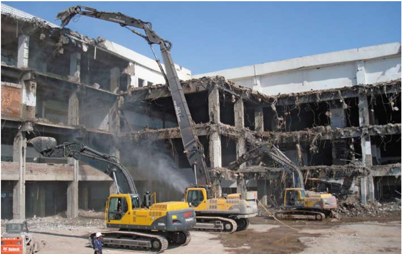
Demolition of T2A Terminal at Mumbai International Airport Ltd using hydraulic crushers.
