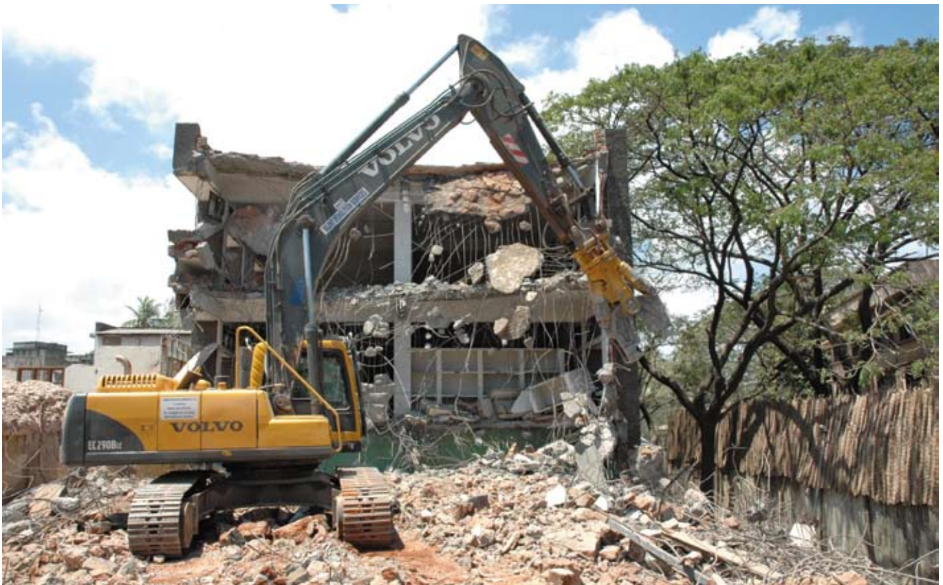
Demolition of low rise structures using normal hydraulic excavator fitted with hydraulic crushers.
