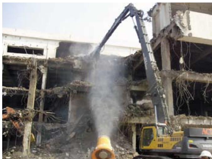
Demolition of high rise building using specialized high reach machine. Special water spray machine used for dust control
